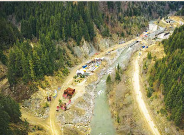
Just one third of the world's rivers remain free-flowing. Dams are the primary barrier to freshwater connectivity. Here, a dam is under construction on the emblematic river Bâsca Mare, Romania, found in the heart of the Carpathian ecoregion of Europe. © Leeway Collective / Balkan River Defence, Courtesy Calin Dejeu
